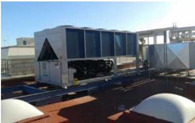
Picture 11. New cooler in boarding module A in Palma de Mallorca
